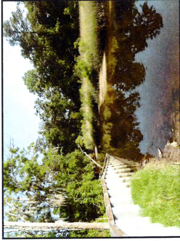
Exhibit 10. Collapsed Sheetpile Wall (4/27/2014)
