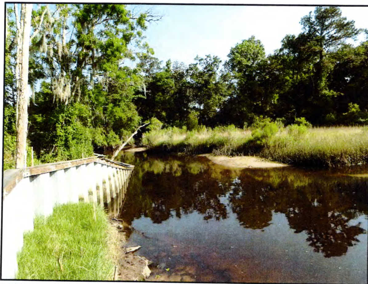
Exhibit 8. Collapsed Sheetpile Retaining Wall (4/27/2014)
